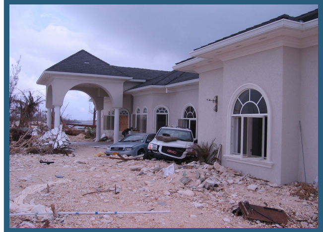
This ICF home in the Cayman Islands withstand the Category 5 devastation of Hurricane Ivan (2004)
